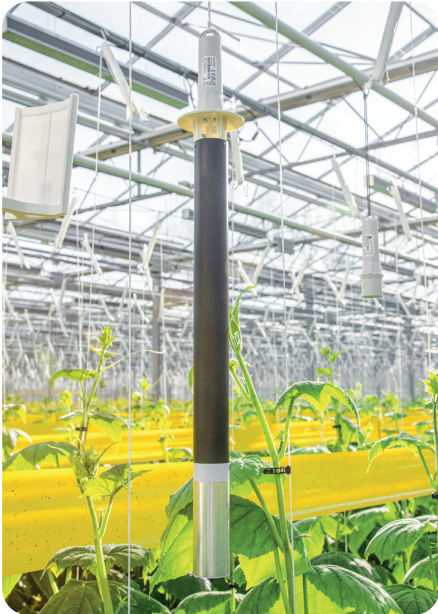
T/RH sensor with Radiation shield installed in the greenhouse.
