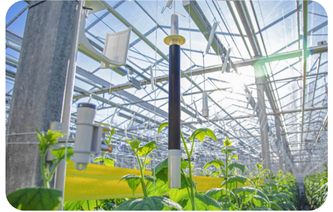
Make data-based decisions to adapt heating and ventilation systems, or sun shading screens according to the plant needs.
