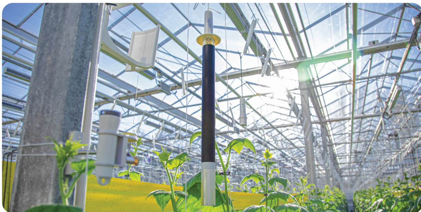
Example of PAR, T/RH with a Radiation shield, and CO 2 sensors installed in the greenhouse to monitor ambient conditions
