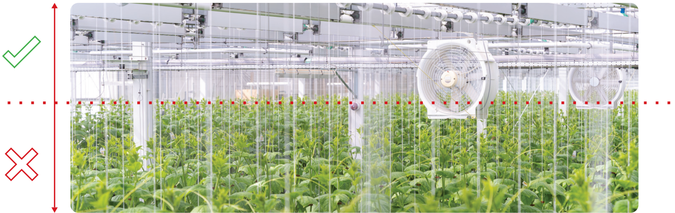
Example of the Base station installed above the tomato plants in the greenhouse.
