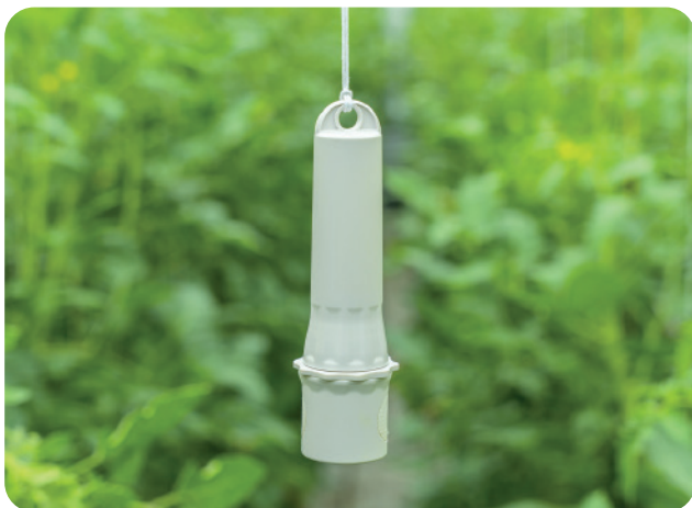
CO 2 and Temperature sensor installed in the greenhouse.
